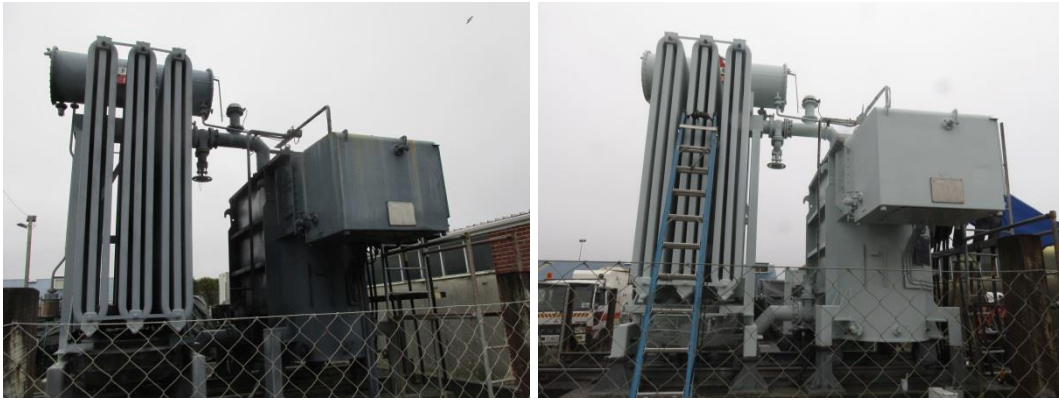
Figure 7-5 Strategic Spare Power Transformer, Pre (Left) & Post (Right) Refurbishment
