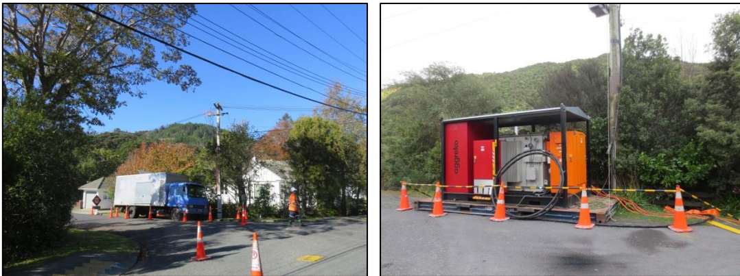
Figure 6-11 Examples of Generators Supporting Planned Work
