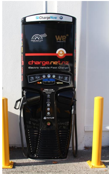
Figure 9-10 Public Electric Vehicle Charger (Upper Hutt)
