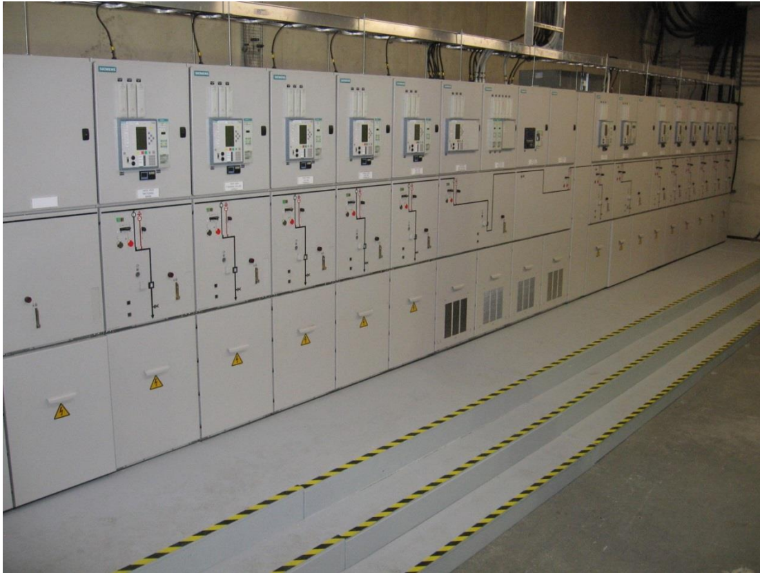
Figure 7-10 11 kV Circuit Breakers at The Terrace Zone Substation
