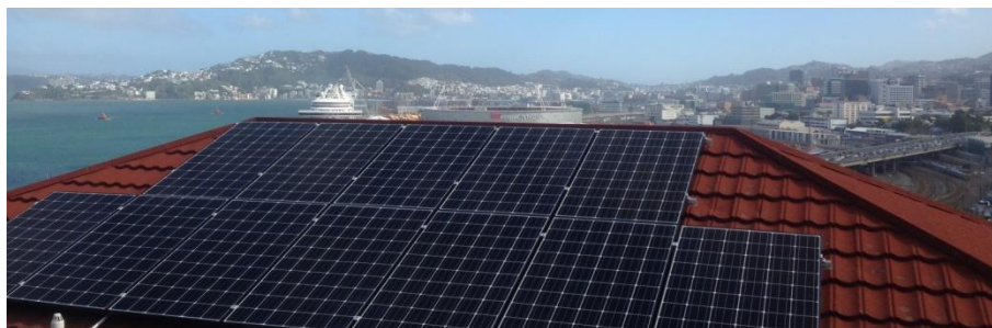
Figure 9-12 A Typical Rooftop PV Installation
