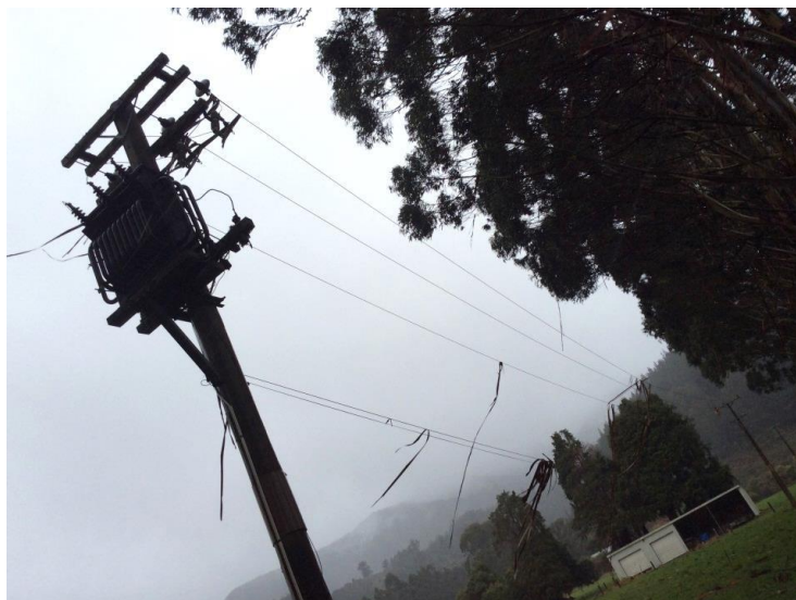
Figure 6-14 Bark Blown onto Overhead Conductors
