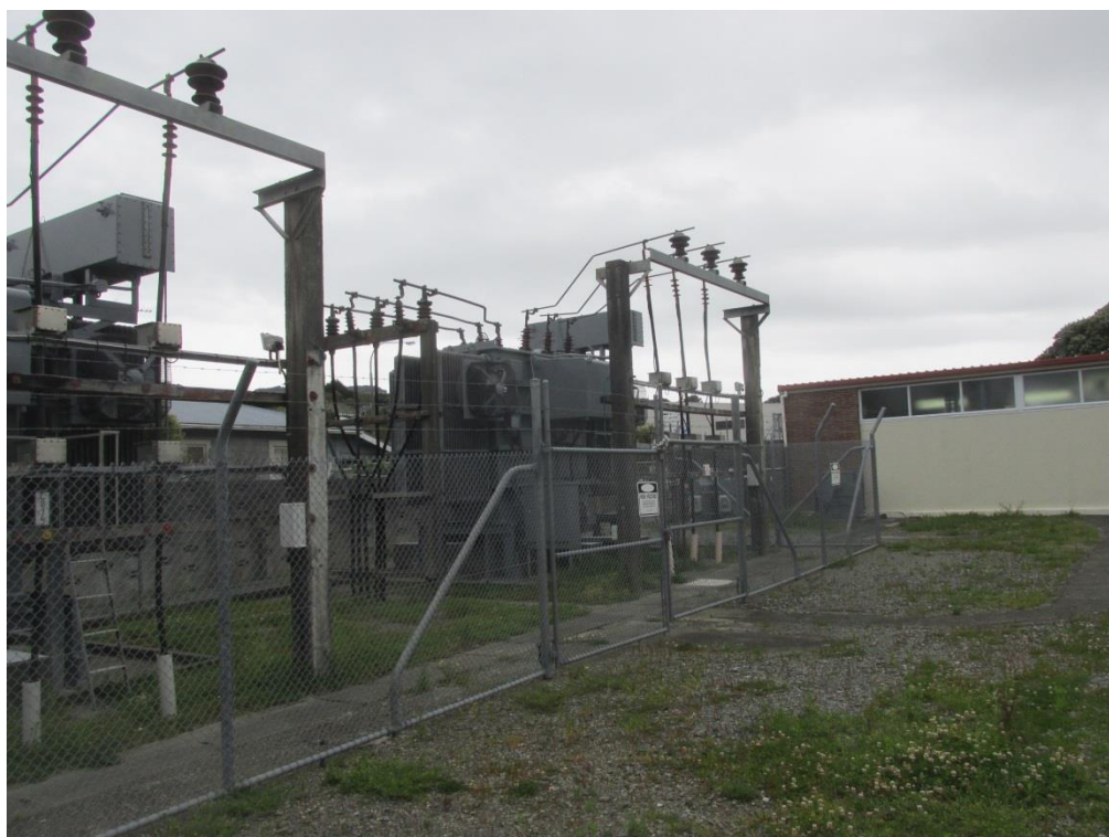
Tawa Zone Substation Power Transformer
