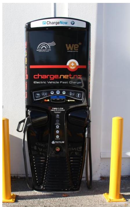
Public Electric Vehicle Charger (Upper Hutt)
