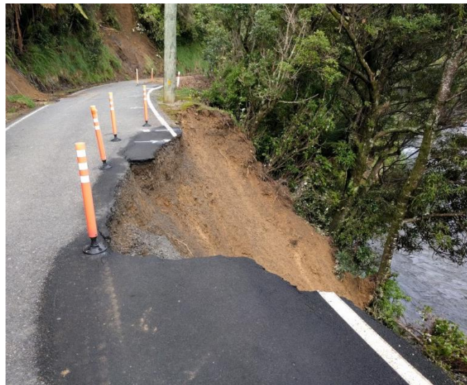
Road Damage and Proximity of WELL pole (Field Test Site)
