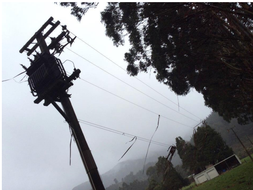
Bark Blown onto Overhead Conductors
