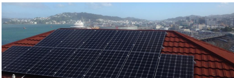
A Typical Rooftop PV Installation
