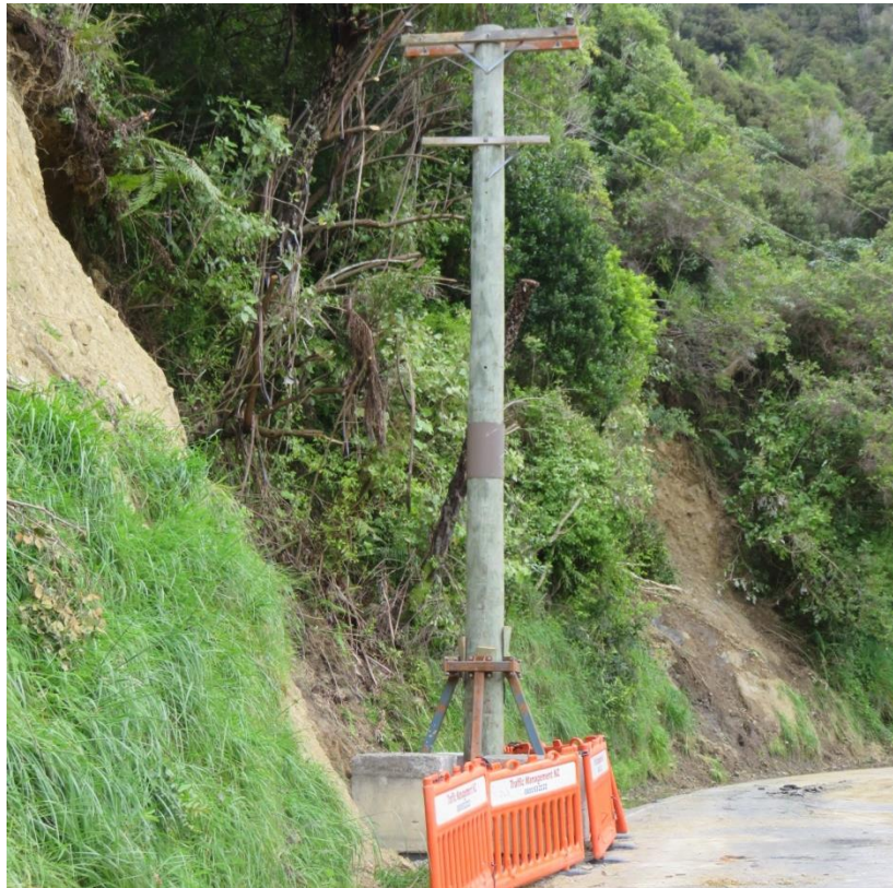
Above Ground Pole Foundation
