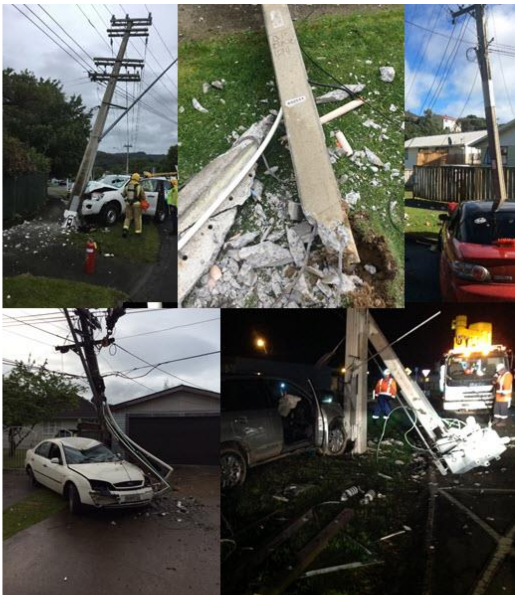
Fault Cause – Car versus Pole
