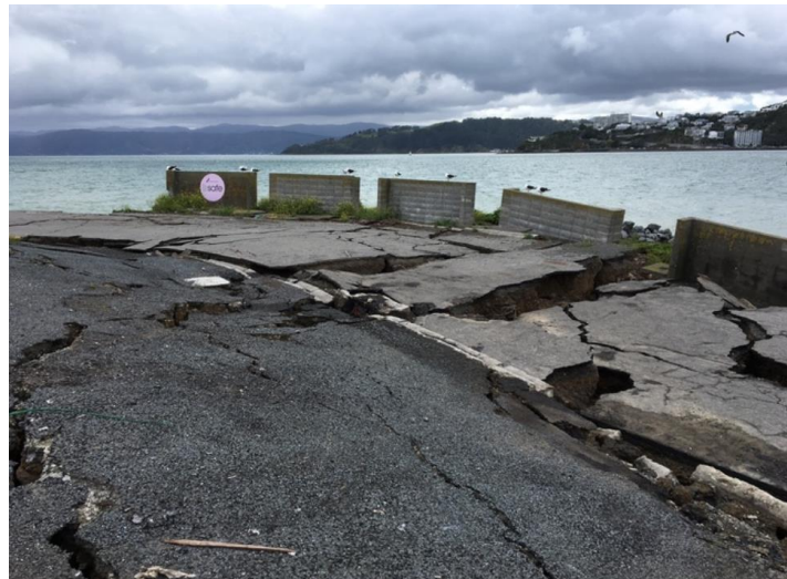
Figure 11-5 Cracked concrete at Wellington's port 70
