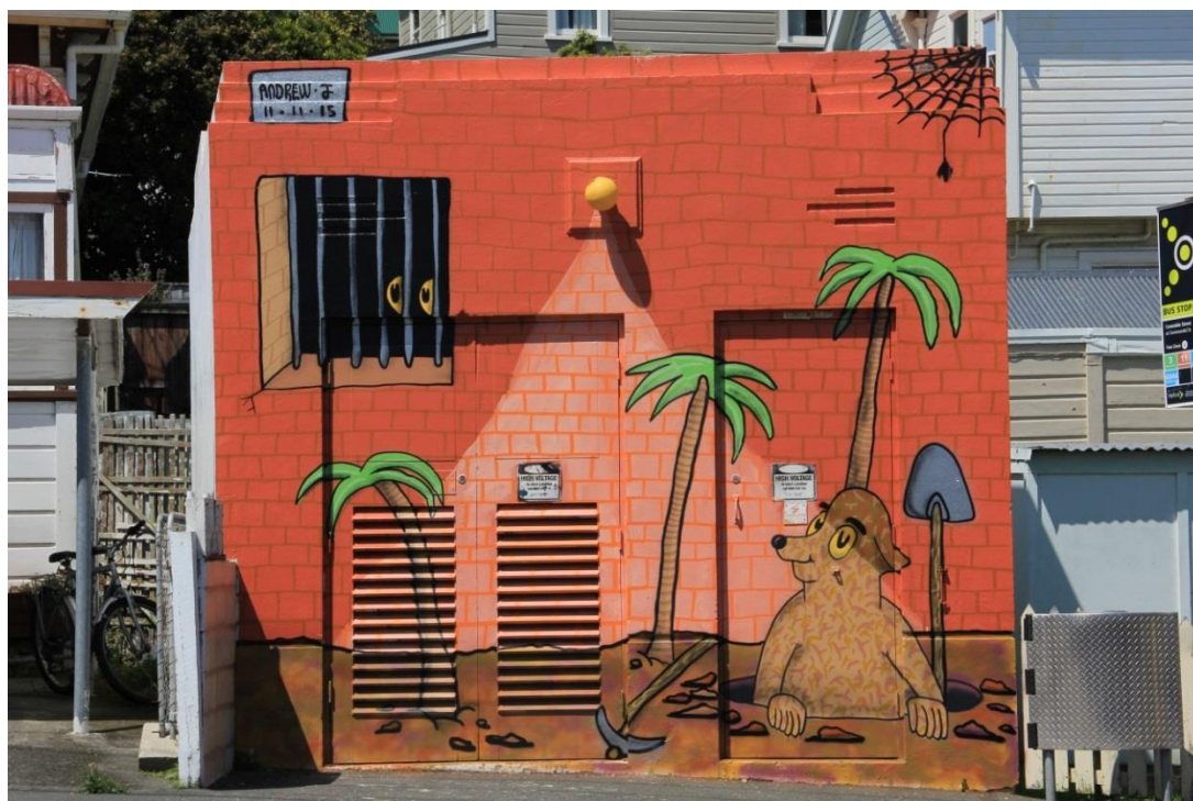
Anti-graffiti Mural on Kiosk Distribution Substation
