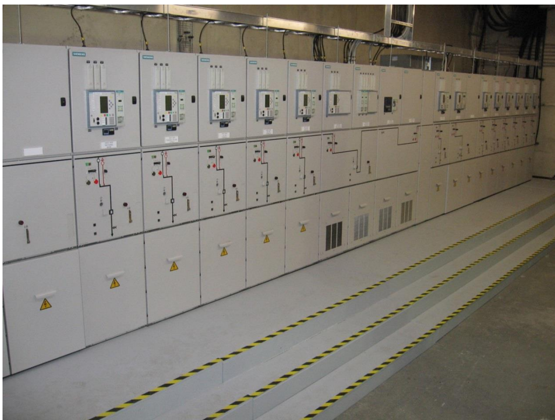
11 kV Circuit Breakers at The Terrace Zone Substation
