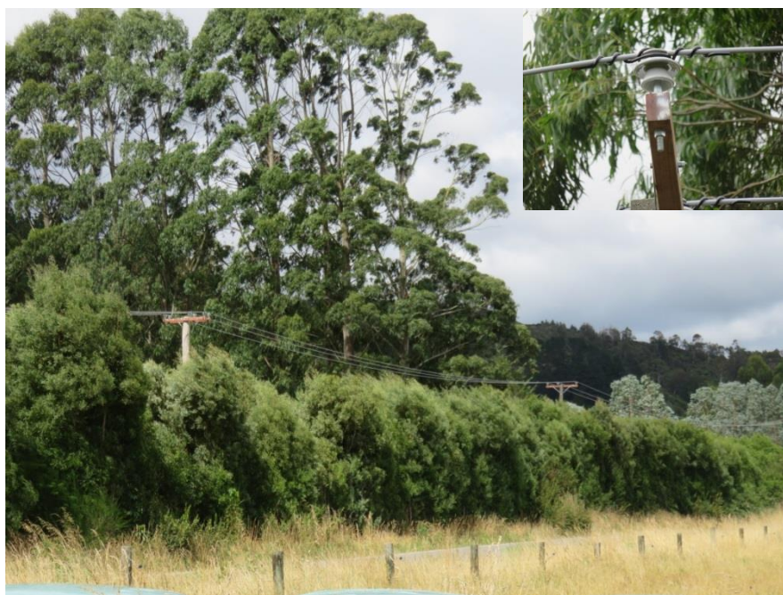
Covered Conductor Trial Installation
